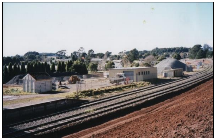
State Rail Contractors – View from south of the line, large heaps of ballast, bare graded slope
