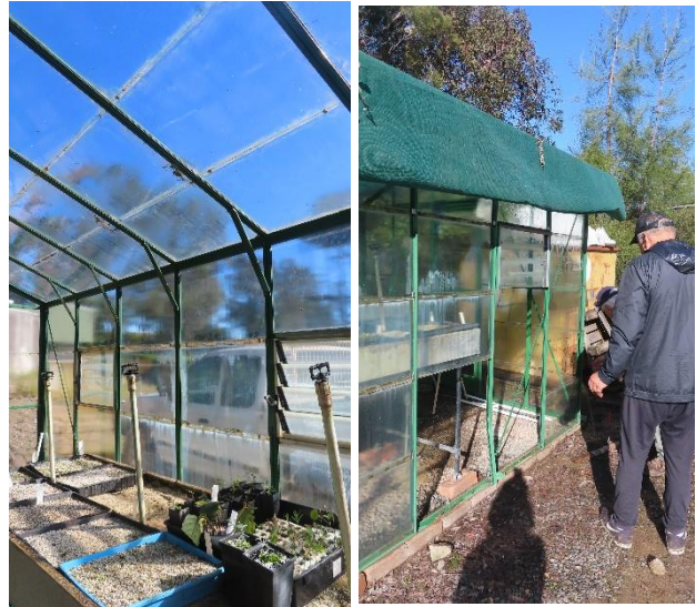
All clean on left but damaged panes removed on right.
