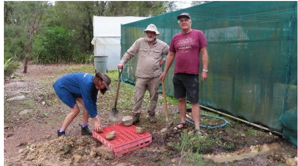
Team with newly constructed tadpole pool. Note woman working and men standing nearby with tools. P Forbes.
